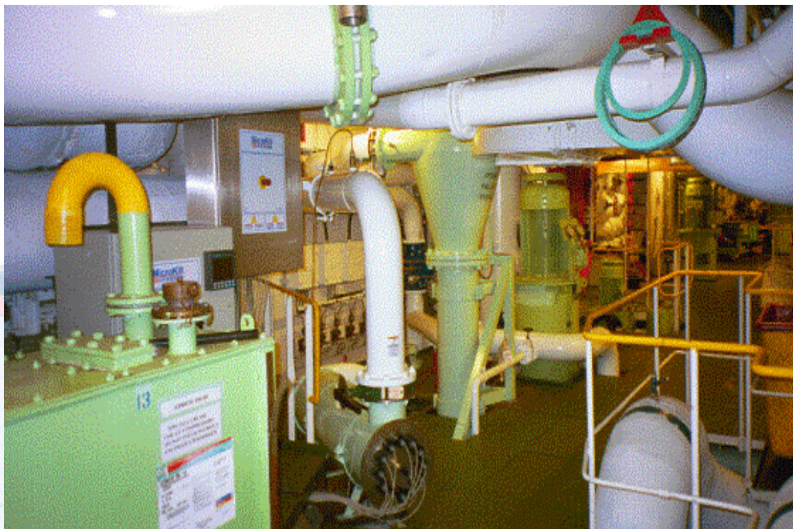
OptiMar Ballast treatment system (cyclon + UV) aboard the "Regal Princess" (photo: http://www.optimarin.com/ )
