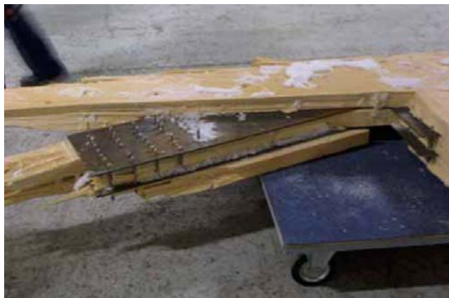
Figure 6. Collapsing of an exhibition hall in Jyväskylä due to missing dowels in one of the joints (Jyväskylä 2003).
