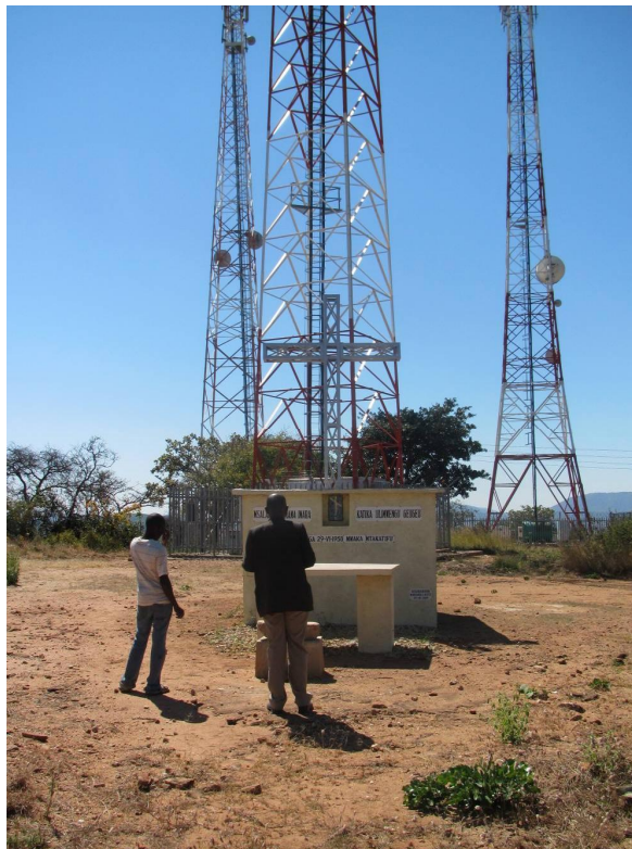
Figure 10. Three base stations on top of a hill in Ipamba. At the front, the altar used in religious ceremonies that are organised on the hill top.
